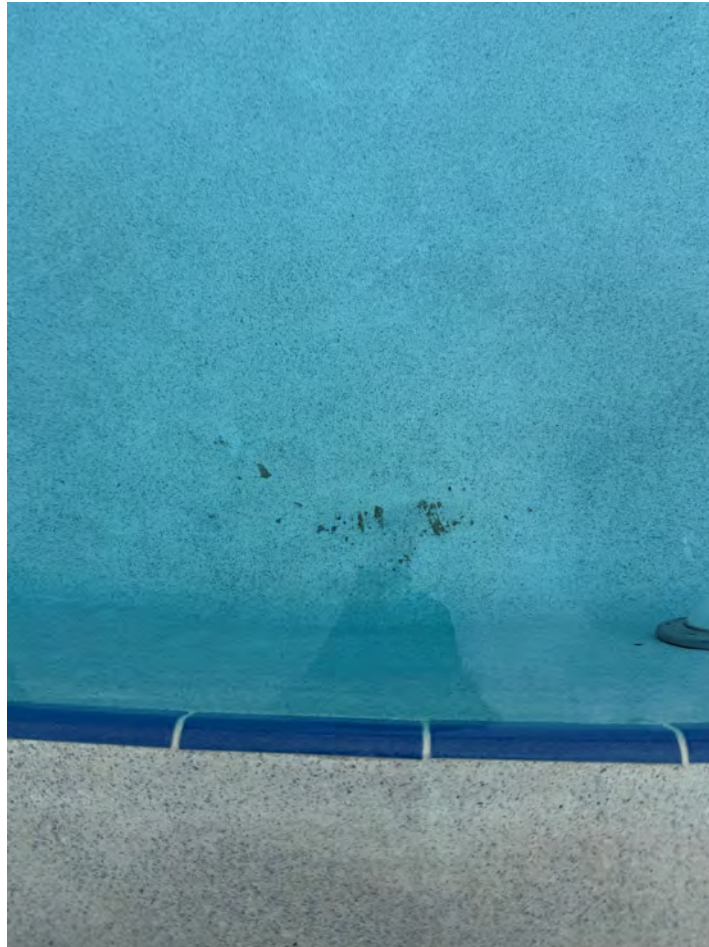
Area where the Diamond Brite finish has worn away
