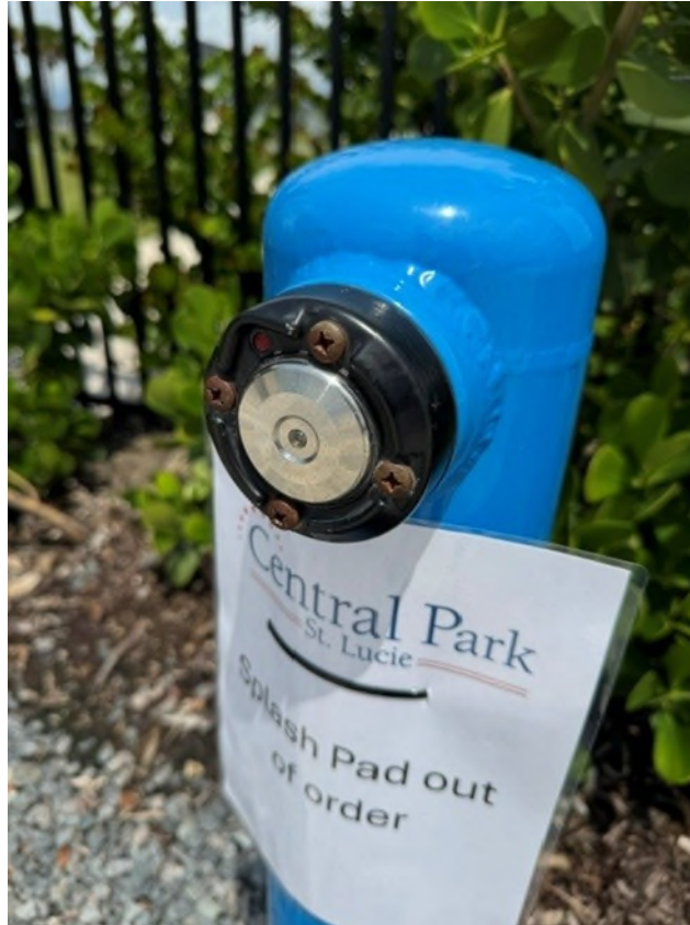
Failed splash pad activation button
