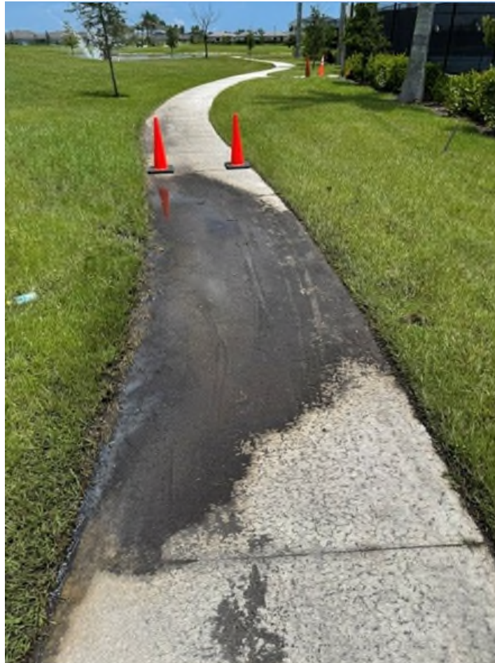
Potential sidewalk slipping hazard marked with cones
